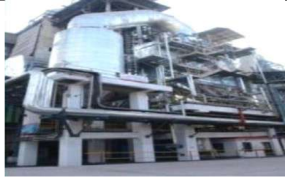
Photo-4- Waste heat recovery system
