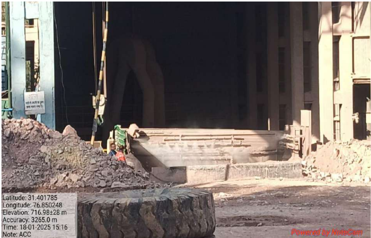
Automatic Mist Fog Dust Suppression System in Unloading area
